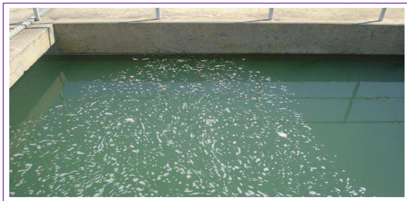
Figure 9 : Bassin de flocculation.
